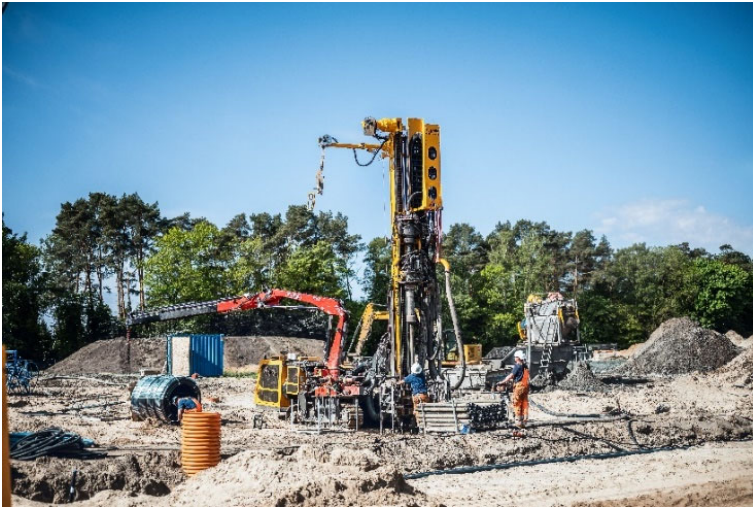
(1) BAUER Resources is installing 135 geothermal probes with an exceptional drilling depth of 170 m.
